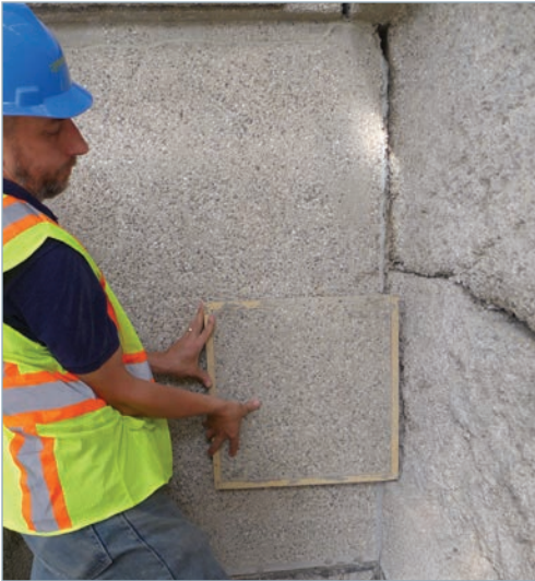
Unity Temple, sample of desired exterior concrete finish compared to existing conditions.
