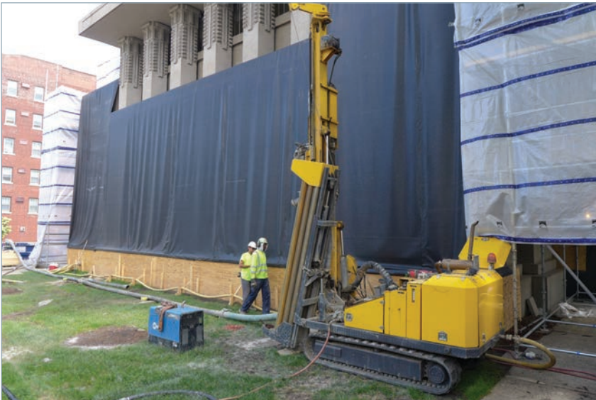
Unity Temple, view of Unity Temple wing and draping of work area during restoration efforts.
