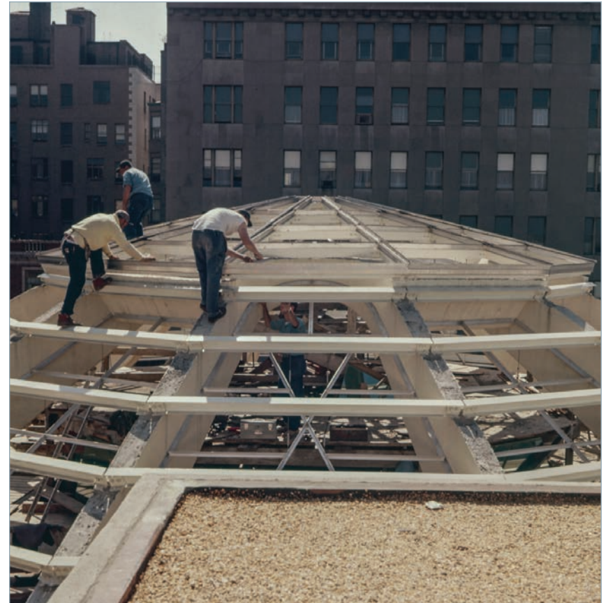
Solomon R. Guggenheim Museum, view of installation of skylight glass, ca. 1956 - 1957. Photograph by William Short. Courtesy of the Solomon R. Guggenheim Foundation.
