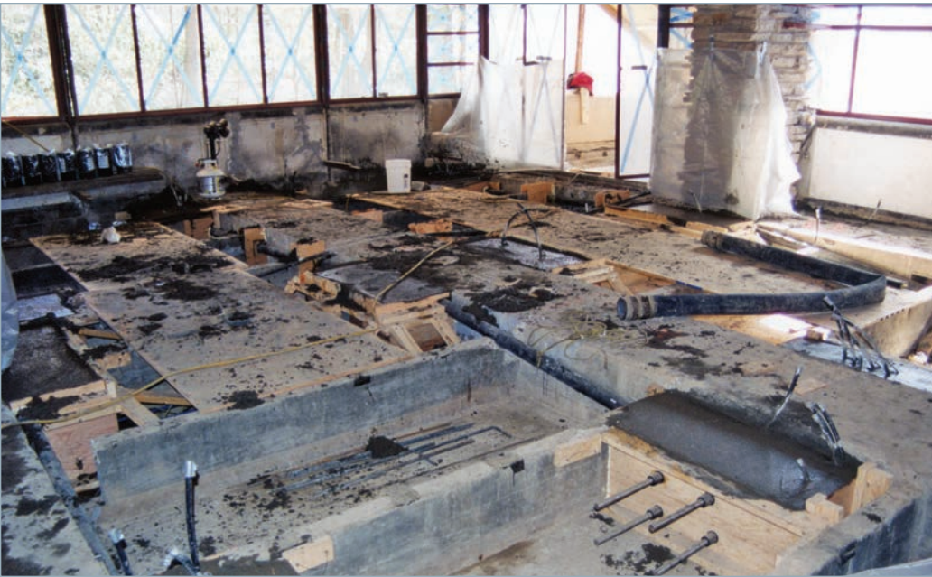
Living room floor reinstallation at Fallingwater, 2002, view of cable channel anchors following concrete pouring. This work was completed as part of an overall preservation effort to slow the deflection of the house's terraces. Structural monitoring of the terraces in 2013-2014 has proved the post tensioning cable installation beneath the living room floors a success. Photograph courtesy of Fallingwater and the Western Pennsylvania Conservancy.
