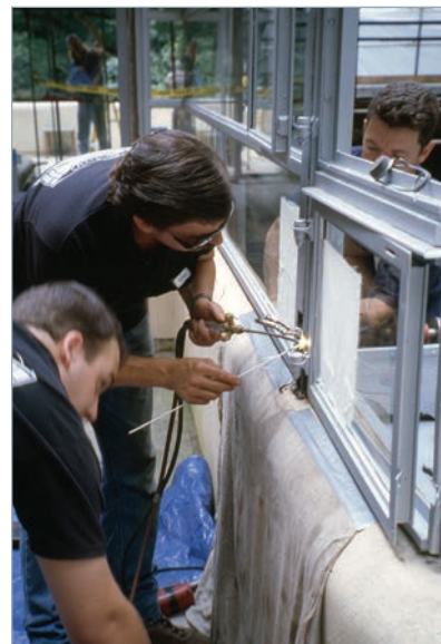
Steel window conservation along the exterior walls of the living room hatch at Fallingwater, September 2001. The steel sash conservation is ongoing, with each window and door frame monitored for corrosion. The paint layer is removed, the steel frames repaired, and an ultraviolet light-filtering glazing replaced. Photograph courtesy of Fallingwater and the Western Pennsylvania Conservancy.
