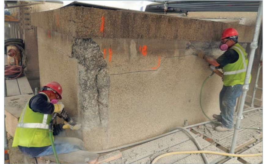
Unity Temple, removal of degraded exterior concrete finish during restoration of building's exterior to historic appearance.
