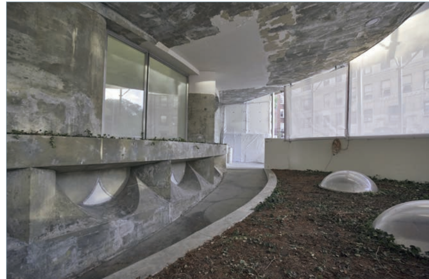
Façade with paint removed during preservation of the Solomon R. Guggenheim Museum, 2005. The preservation effort removed eleven layers of paint from the surface, resulting in a revelation that Wright's original pigment was a light-yellow "buff" shade, used only until the early 1960s. The color became more off-white or gray over time, and in the end, the museum was painted off-white, the hue most associated with the building's history. Photograph by David Heald, courtesy of the Solomon R. Guggenheim Foundation.
