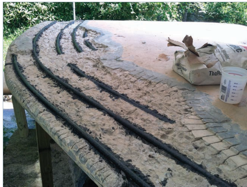
As part of ongoing preservation of Fallingwater, the concrete step canopy of the stairs leading from the main house to the guest house was repaired following cracking and material loss in June 2013. The work provided insight into the concentric arrangement of the canopy's reinforcing system, shown here after treatment with an anticorrosive agent. The concrete was reapplied and the rolled edges of the canopy formed by hand before applying the finish paint coat. Photograph courtesy of Fallingwater and the Western Pennsylvania Conservancy.
