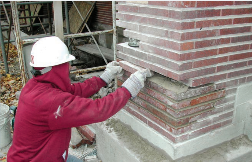
Installation of salvaged bricks on the south façade of the Frederick C. Robie House, November 2002. The replacement bricks were used in areas where missing and or severely damaged bricks were found, in this case on a pier on south façade of building.
