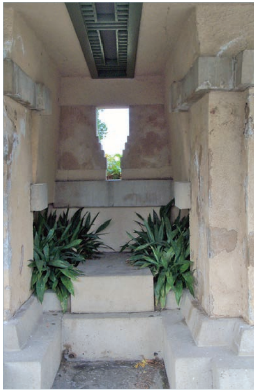
Preservation of the loggia near the entrance to Hollyhock House was completed to investigate surface cracks in the concrete stucco exterior as well as any possible structural problems. Once completed, the surface was repaired and plastered and covered with a coat of paint. Photograph by Jeffrey Herr, courtesy of Hollyhock House.
