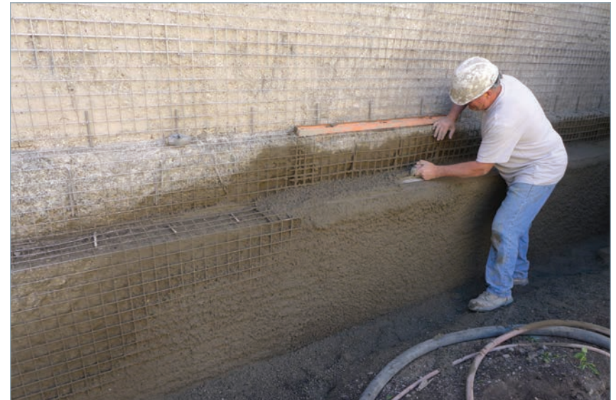
Unity Temple, application of concrete finish to exterior walls where it had been removed due to degradation.
